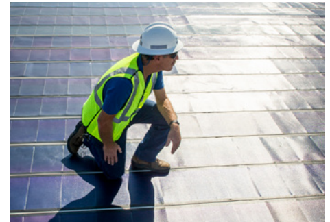
One of the largest thin-film solar installations in the United States, as measured by production capacity, can be found on the roof of Boeing's newest final assembly building at the North Charleston, S.C., facility. (Boeing photo)
